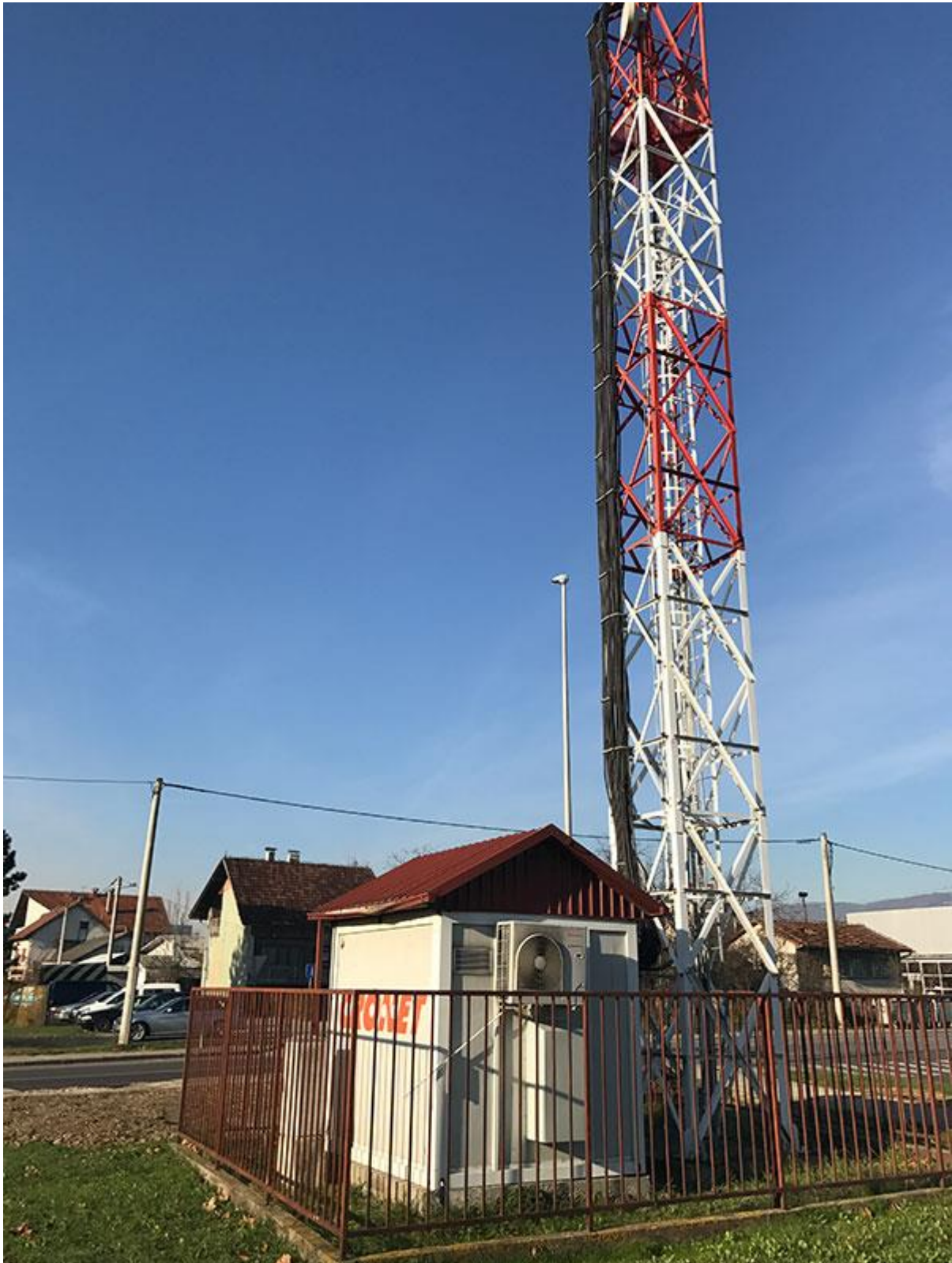
Fig. 1 – Telecommunication base station
