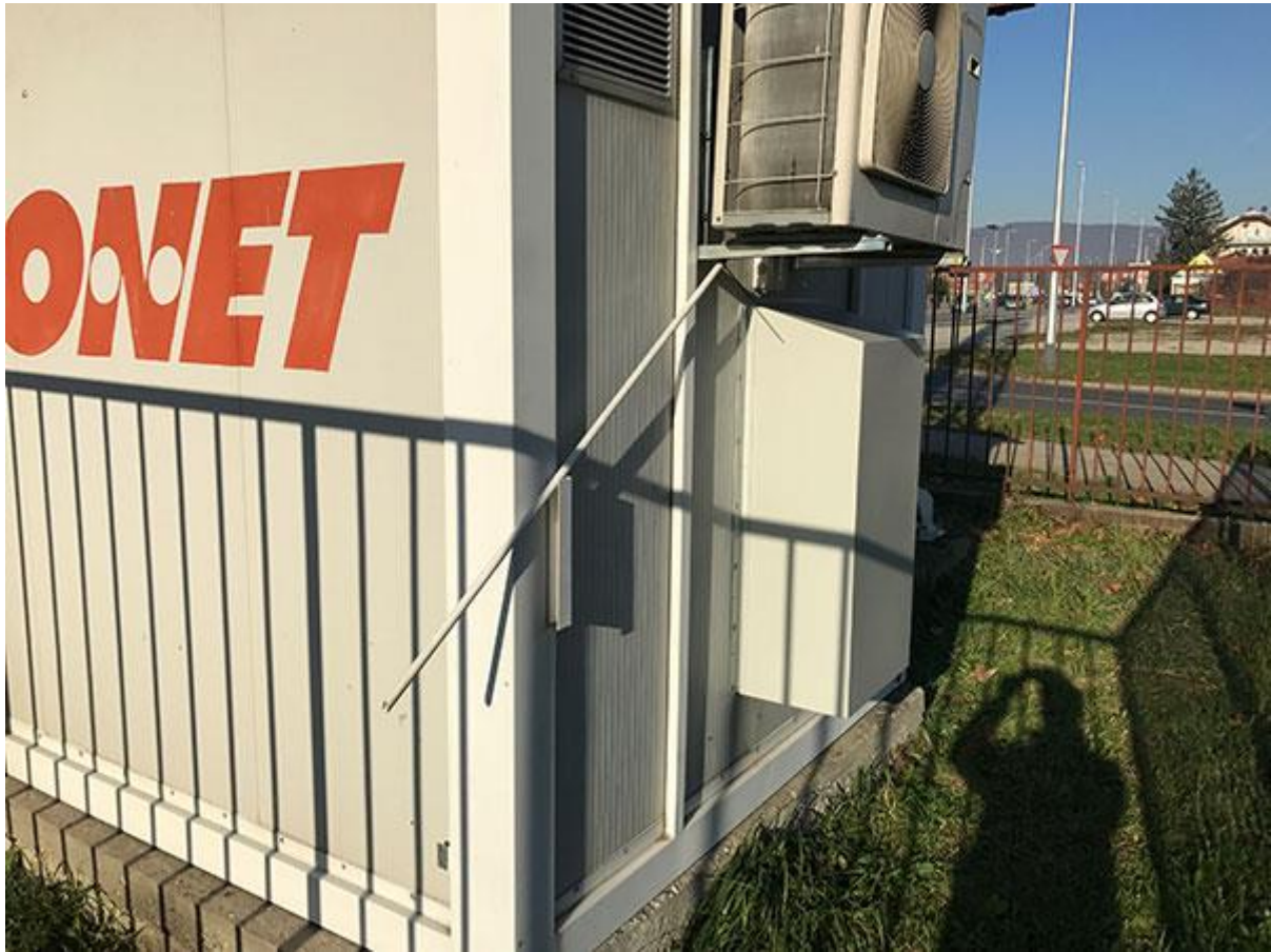
Fig. 4 – Outdoor free cooling unit
